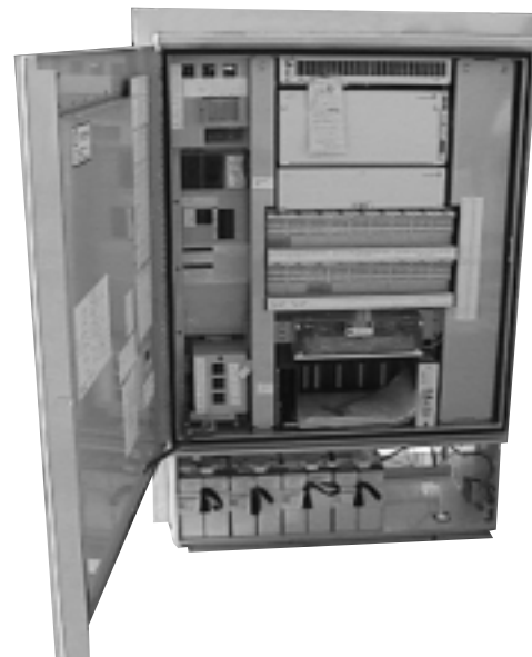
80 Series Cabinet with FA 12-125 Batteries installed
